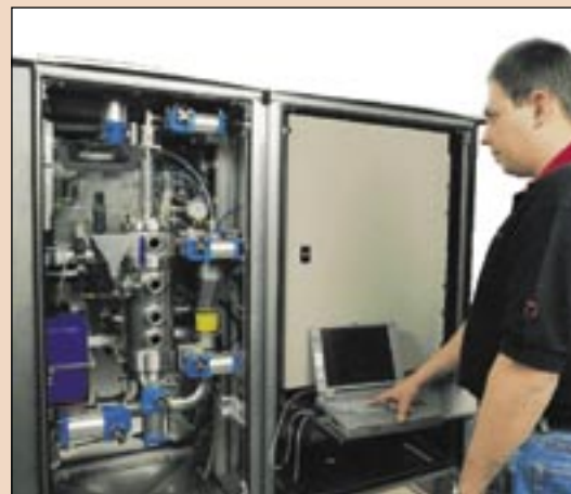
Valves and actuators for analyzer.
